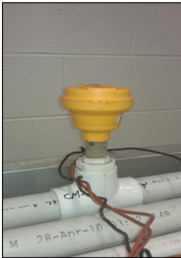
Figure 44: Electrical conductivity meter
