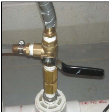
Figure 47: Three-way valve and check valve
